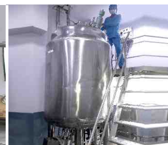
LIQUID MANUFACTURING PLANT
